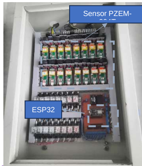
Gambar 6. Panel Utama Laboratorium Mekatronika
